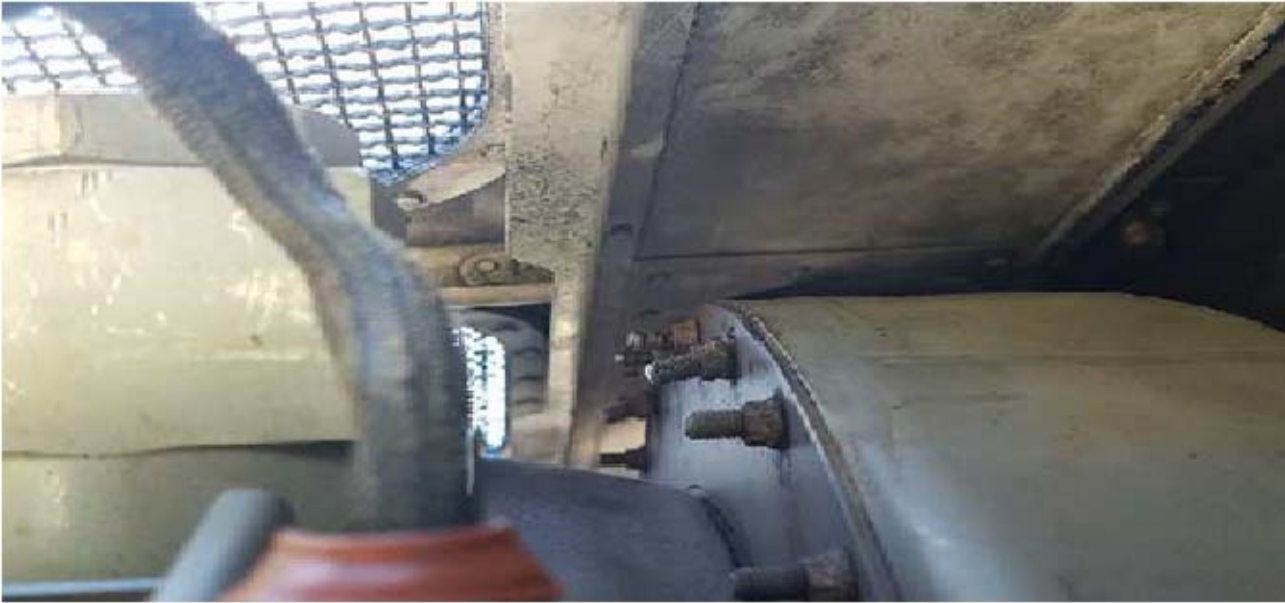
Example of Broken Compressor Diffuser Studs Figure 1
