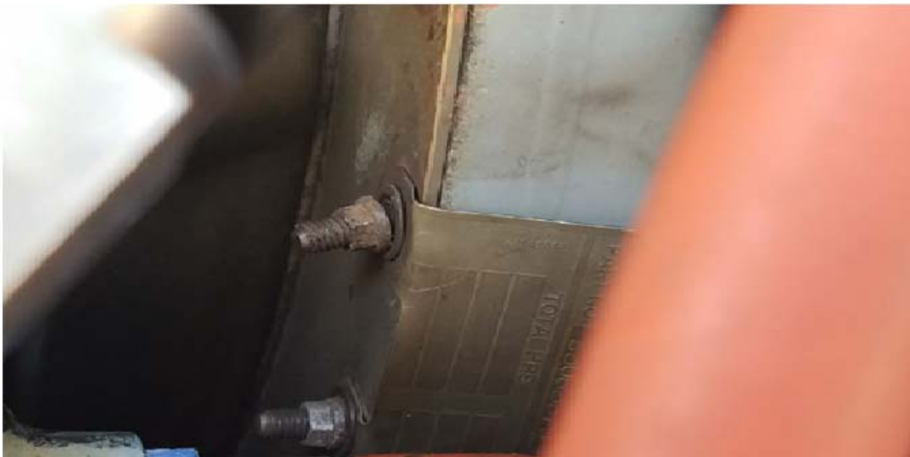
Example of Broken Compressor Diffuser Stud Figure 2
